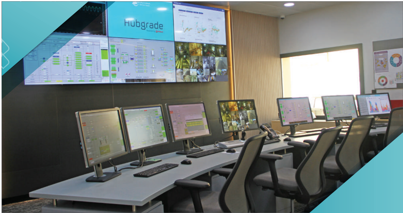
Figure 4: Upgraded Control Room & Hubgrade Centre
